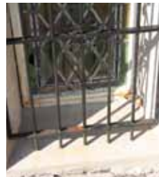
These photos depict several of our restoration project needs.
